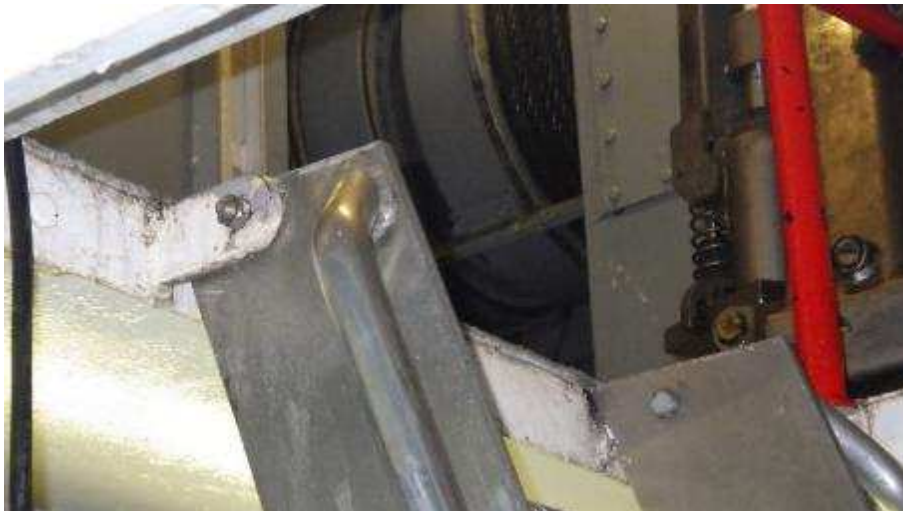
Figure 6– View from the stairs leading to engine room equipment
