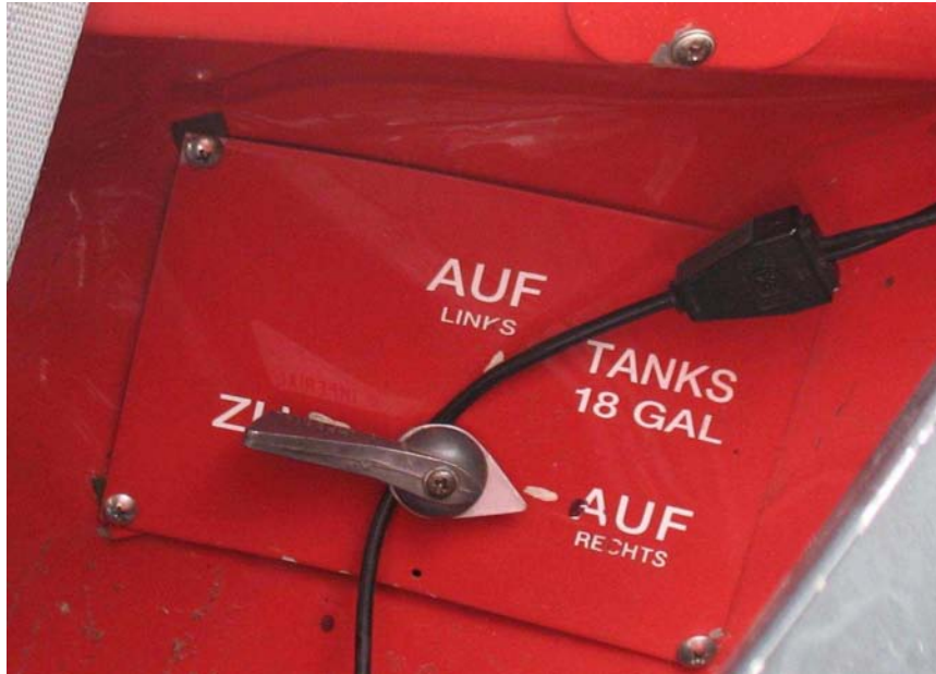
Fuel Tank Selector Valve (on D-EFXY)
