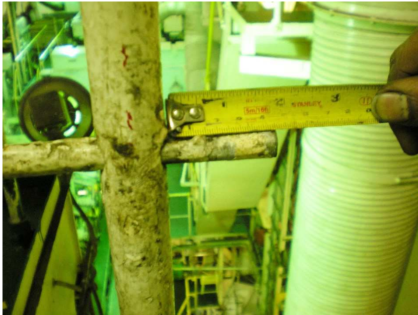
Figure 9 - Broken tack weld allowing for 30 mm horizontal movement
