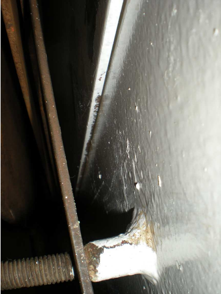
Figure 11 - Threaded rods that holds steel plates in position
