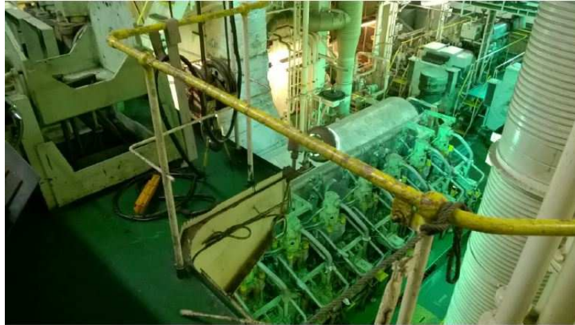
Figure 6 - Lower part of railing (loose) where crewmember fell onto
