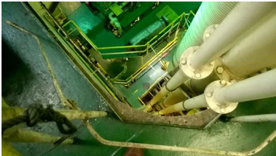
Figure 3 - Downward view of engine from platform
