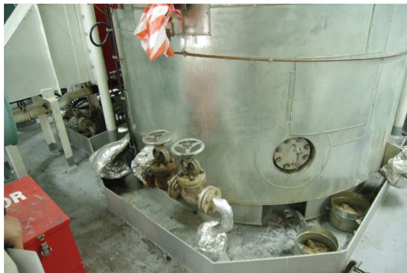
Figure 8 - handhole cover on auxiliary boiler
