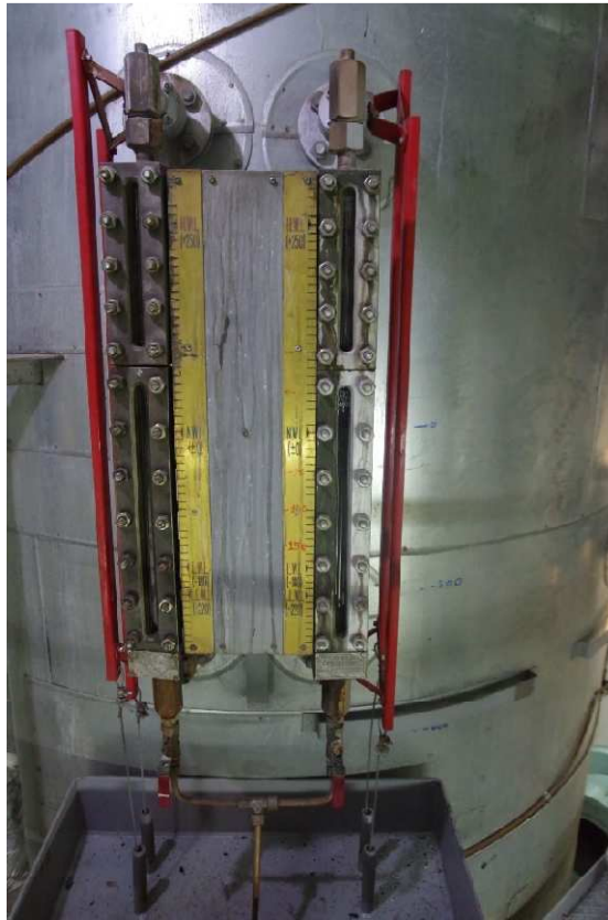
Figure 7 - glass water level indicating gauges
